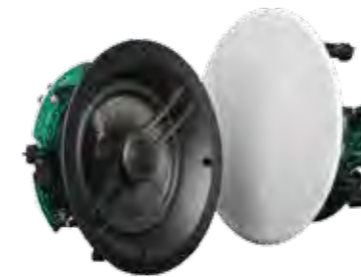
SONOS AMP LOCATED IN THE BEDROOM JOINERY UNIT CONNECTED TO THE AUDIO RETURN CHANNEL (ARC) OF THE BEDROOM TV CONNECTING BEDROOM AND ENSUITE SPEAKERS AS A SINGLE ZONE.
